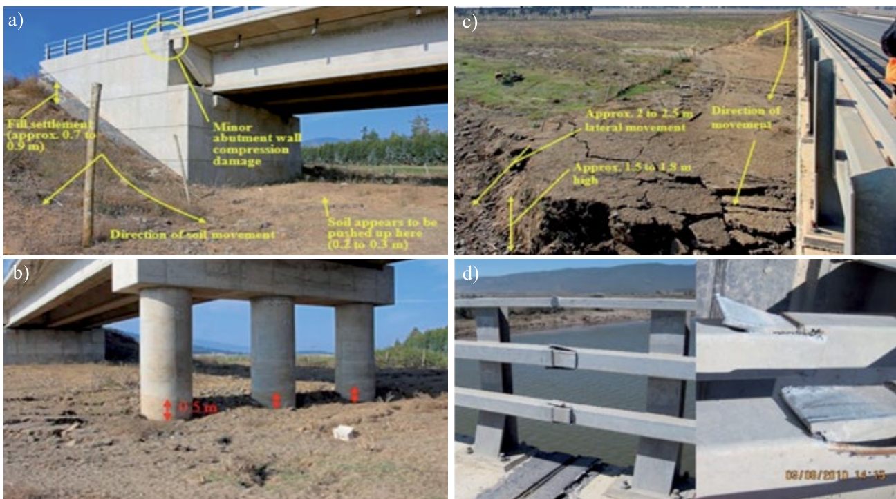
Figure 1: a) North abutment, b) lateral displacement towards the river, c) soil settlement at interior pier at northeast abutment (FHWA, 2011), and (d) handrail failures at the bridge deck
